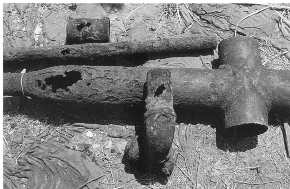
Corrosion of buried pipe.
